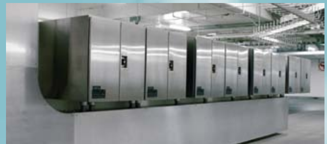
Set Stage Power Distribution Line-up
